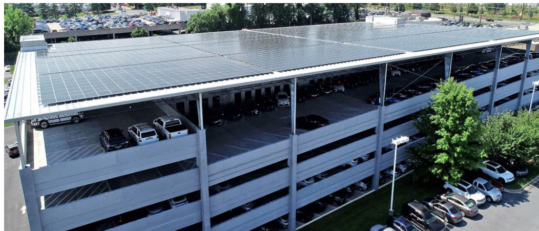
Figure 8. Solar panels installed on parking garages present an opportunity to integrate sustainable features onto transit infrastructure.
