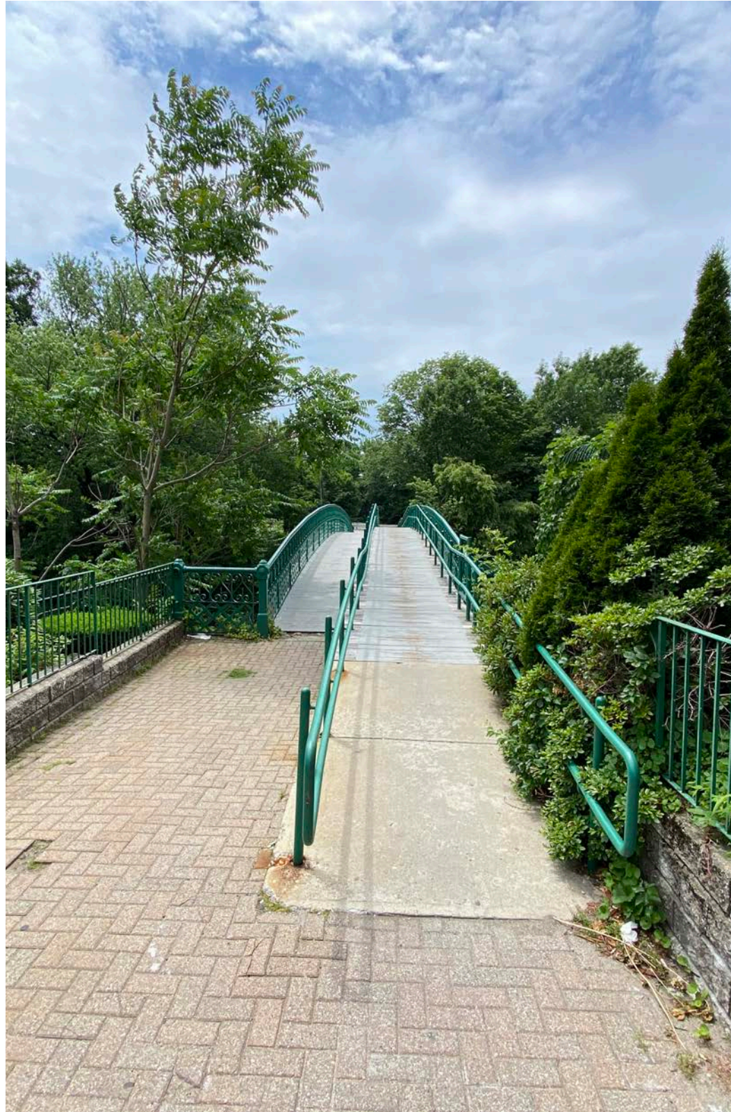
Figure 19. The John D. Hand Memorial Bridge is in need of maintenance and care to restore this historic crossing to its former glory.
