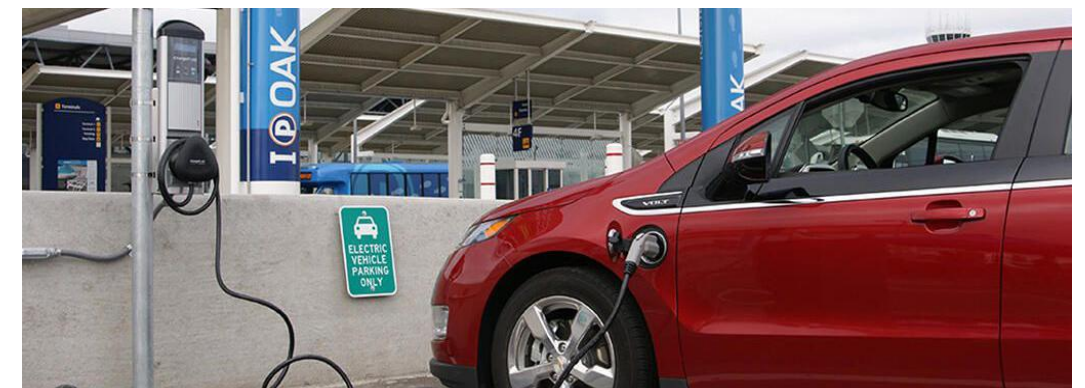
Figure 9. Electric charging stations provide great incentives for increased retail activity, as car charging can take anywhere from 20 minutes to a few hours.
