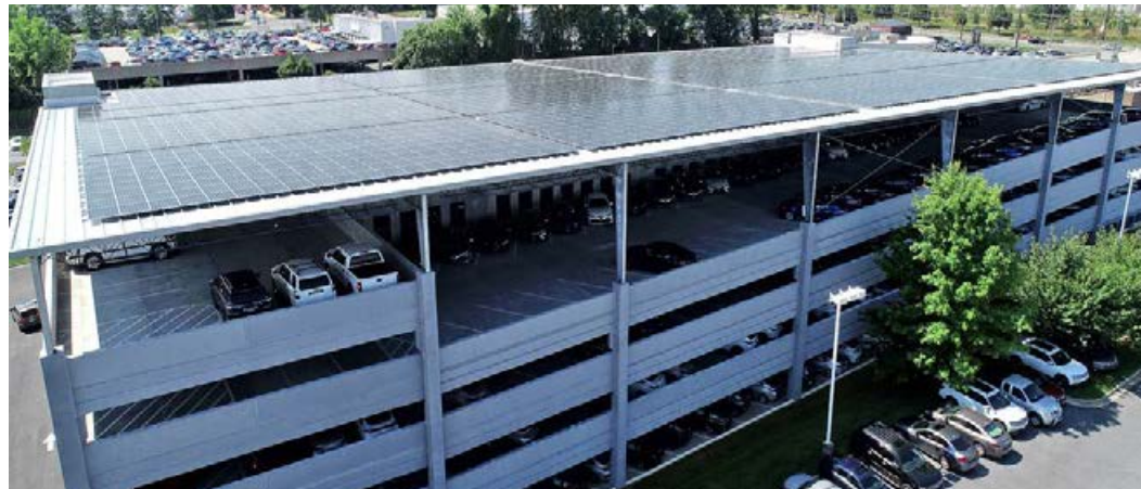
Figure 8. Solar panels installed on parking garages present an opportunity to integrate sustainable features onto transit infrastructure.
